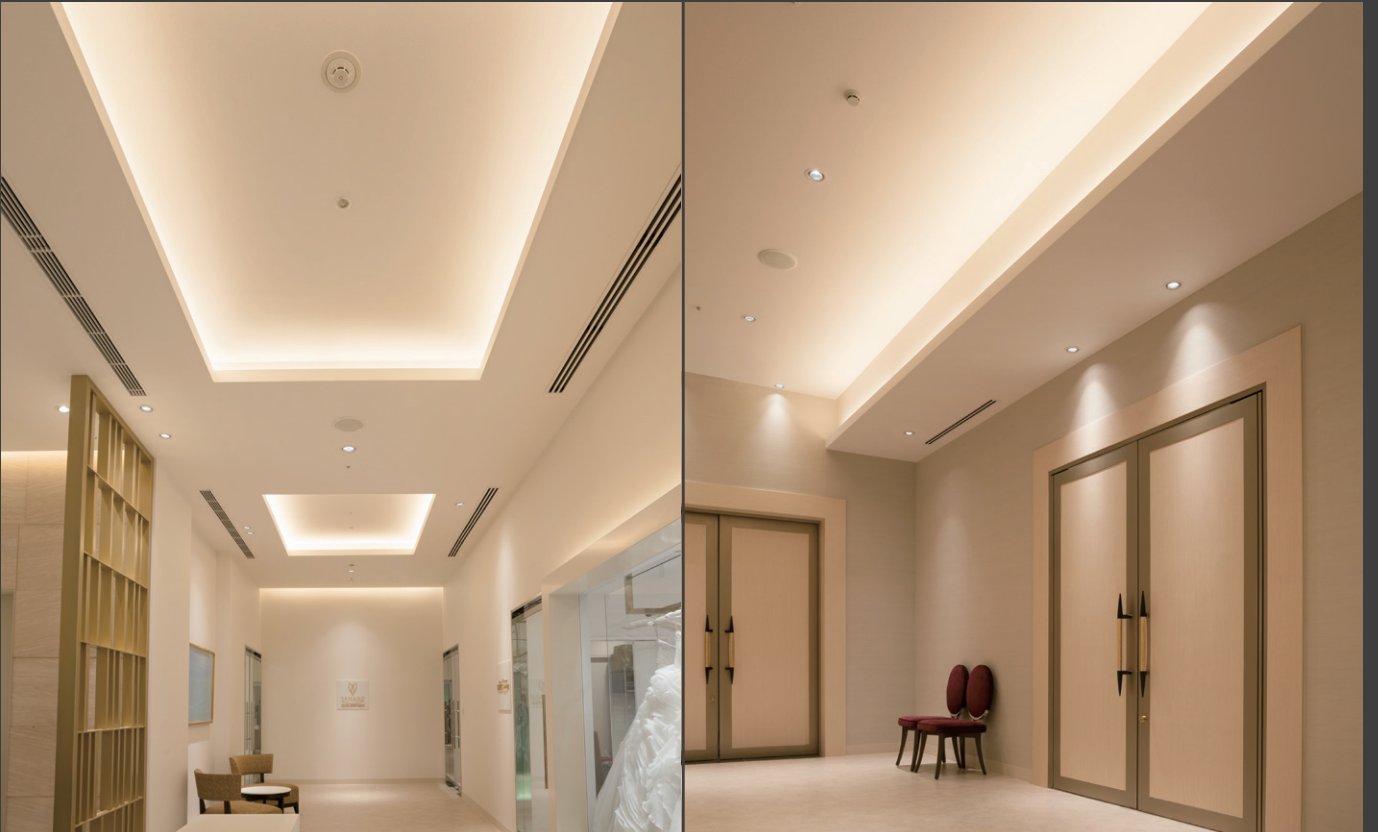
THE WESTIN AWAJI ISLAND RESORT & CONFERENCE CENTER repair work Location: Japan Architect office: J.FRONT DESIGN & CONSTRUCTION Co.,Ltd. Lighting design: KOIZUMI LIGHTING TECHNOLOGY CORP. Construction: J.FRONT DESIGN & CONSTRUCTION Co.,Ltd.
